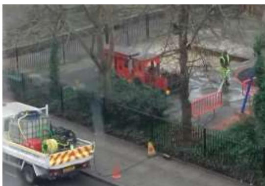
Islington Council workers jet-washing the playground. Note: They are carrying their own water supply.
